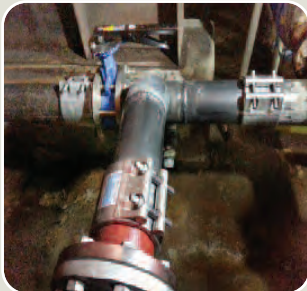
▲ Netherland desalination treatment facilities
