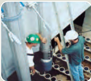
▲ Canada: water purification facility
