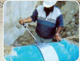
▲ UK: buried water supply pipes
